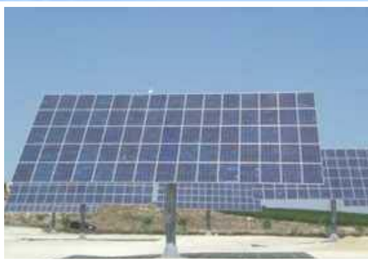
Solar Power Plant / System
