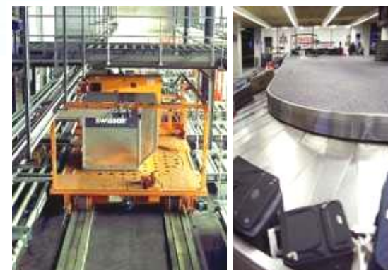
Airport Cargo / Baggage System
